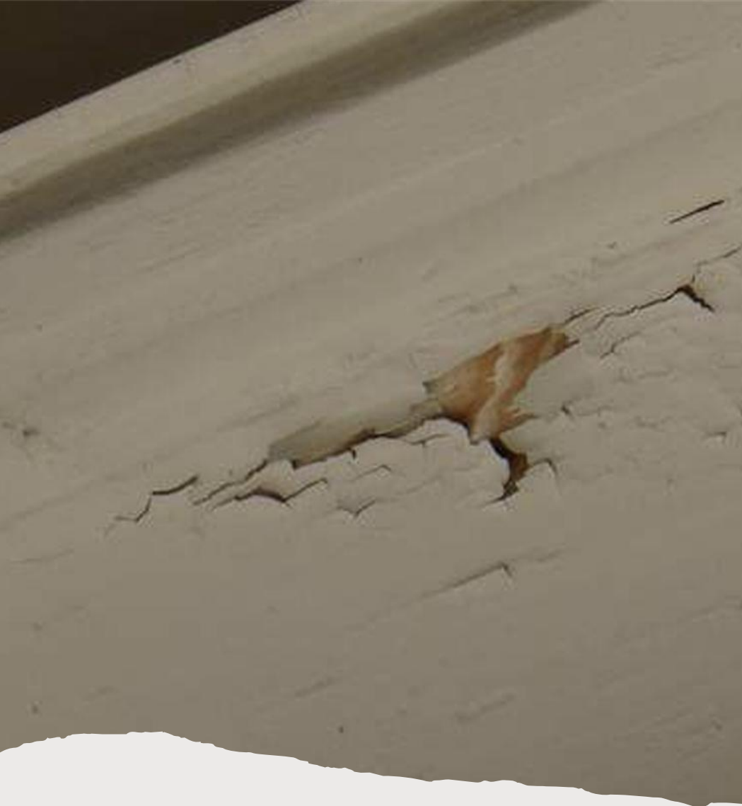
Water damage on wood fascia board, leaking downspouts
